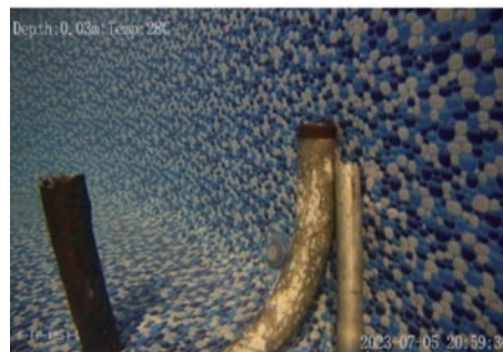
(b) Tape and hole defects
